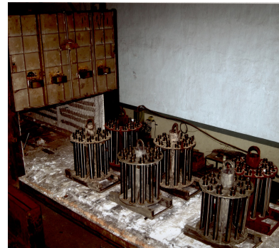
Fig VII: Sleeves in electrical bogie furnace
